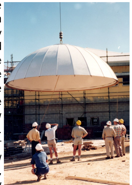
Raising the dome for the Engineering Centre building at CQU . Central Queensland University photograph
